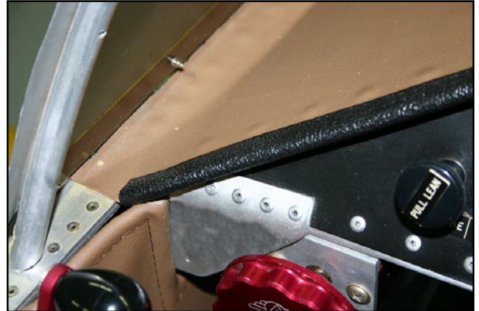
Adding a small aluminum extension to the glareshield allows the glareshield material to be wrapped around the extension and finished with an edge protector.
